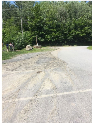
Drainage from road is depositing sediment along the GMVS driveway and parking area.
