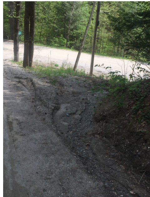
Figure A10. General road and ditch improvements are proposed for the Richardson Rd Lower site.
