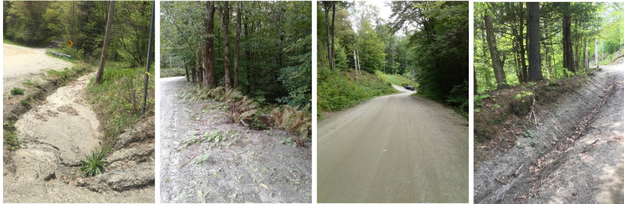
The existing sediment trap at the bottom of Richardson Rd is overwhelmed by sediment and overflowing to Crossett Brook.
