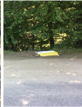
A pavement shim is recommended where water is flowing over bank (see sand bags) instead of designed flow path to bioretention area.
