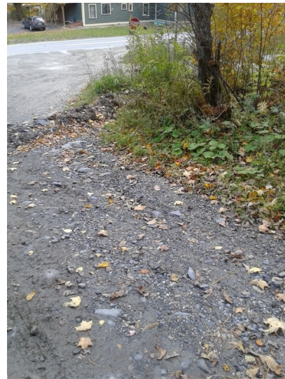
Figure E10. Drainage from the access drive currently drains to a stream.
