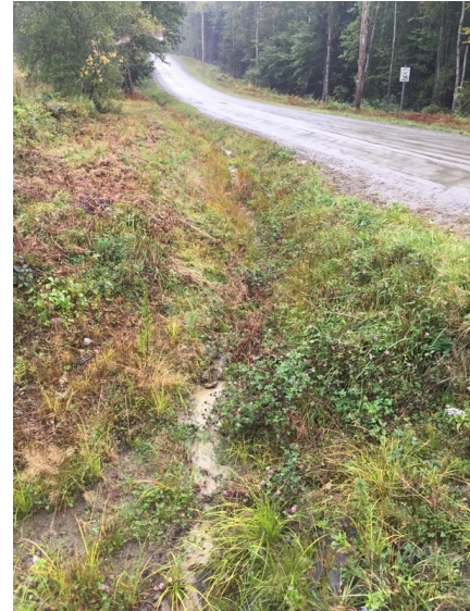
Figure B12. Stormwater within roadside ditch is actively transporting sediment to stream.
