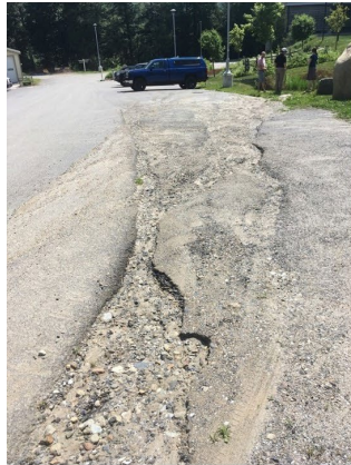
Drainage from the road is causing erosion along the GMVS driveway and in unpaved parking area.
