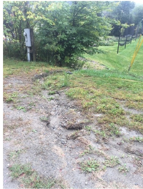
Figure B9. Stormwater is running over Moulton Rd and causing erosion onto GMVS property.
