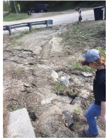
Figure A9. General road and ditch improvements are proposed for the Ward Hill Rd and Route 100 site.
