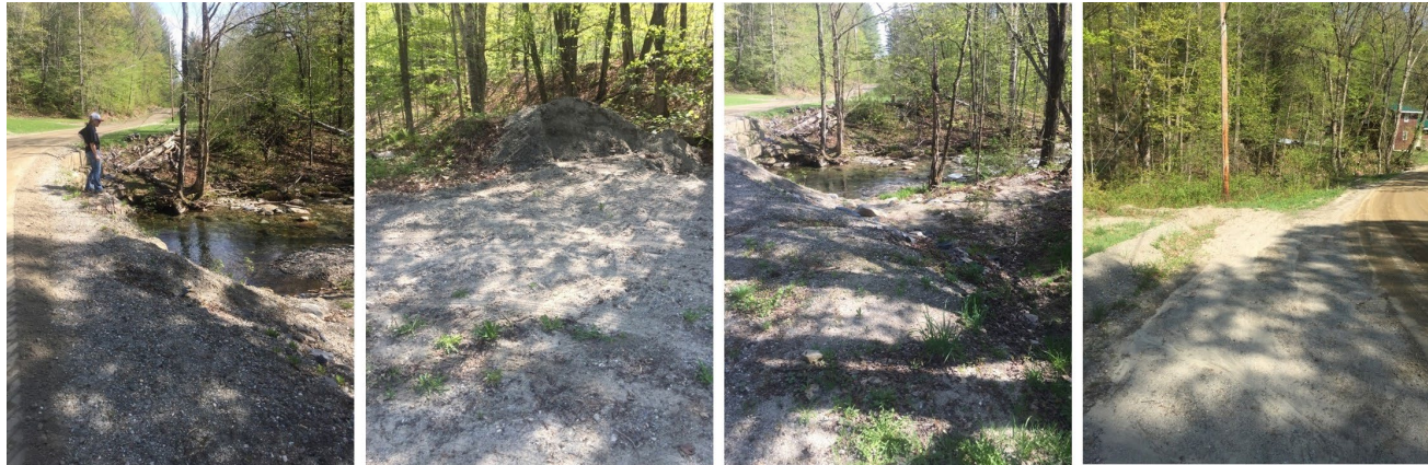
Road drainage is directly connected to Dowsville Brook.
