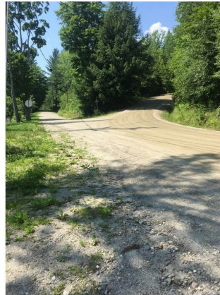
Drainage from Moulton Rd and Glen View Rd is flowing over the road surface to the School's property.
