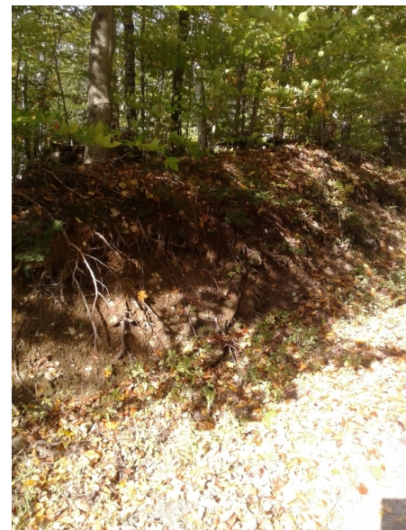
Figure B11. Erosion was noted within roadside ditch and at culvert outlet.
