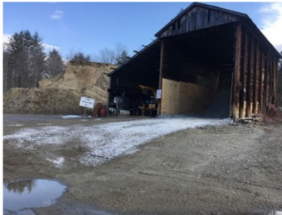
Salt storage at the Town Garage should be improved and any spills cleaned up immediately.
