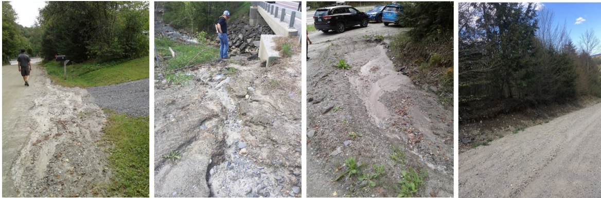
Stormwater is running over the road and depositing sediment where a driveway culvert is not present.
